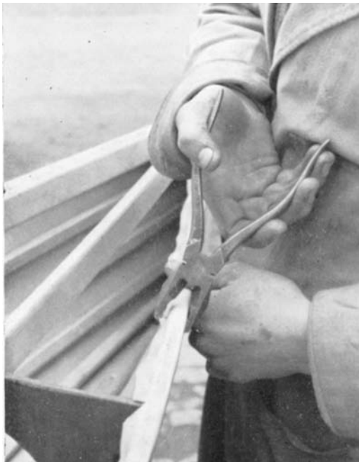
9. Squeezing in tacks with pliers where there is insufficient room to swing a hammer.
